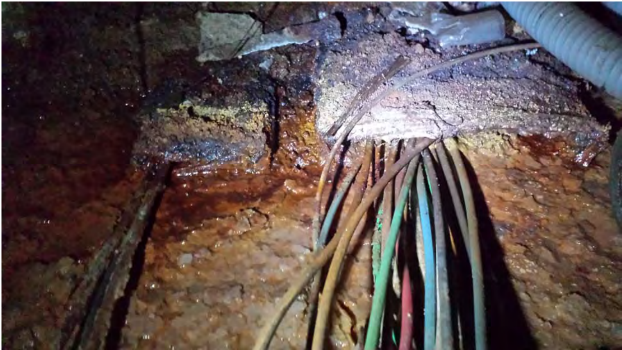
Photo #6 – Condition of Existing Duct inside Kiosk
